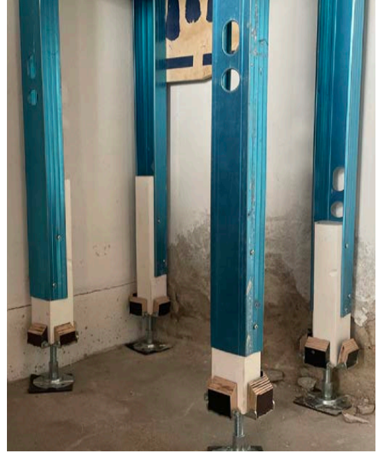
Feet construction on unstable ground
